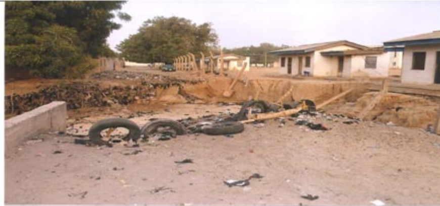
Plate 1: Cut off Road by Gully Erosion behind Mobile Police Barrack
