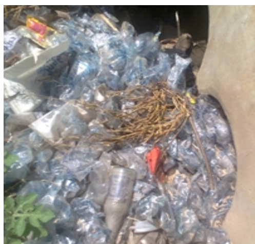
Fig. 5: Blocked Drainage by Waste Polythene wastes in the University Staff Quarters Crescent Line
