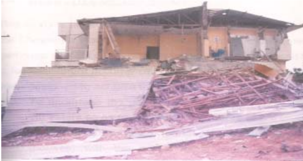
Figure 1: Collapsed House No. 54 at Oba Overanwen Road, Gwarimpa, Abuja
