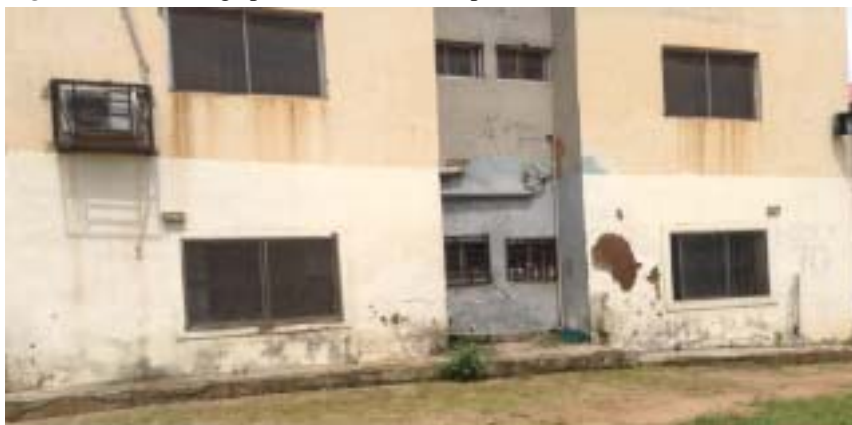
Figure 6: High rise building without drainage in Gwarimpa. Source: Fieldwork, 2015
