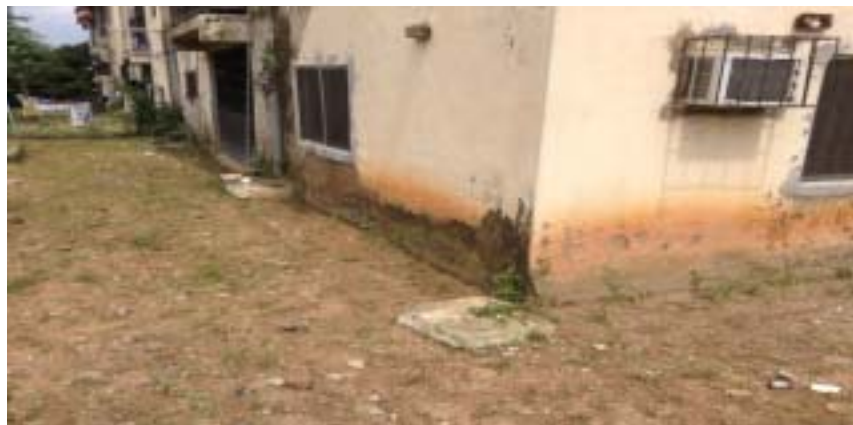
Figure 5: No drainage provision in Gwarimpa Source: Fieldwork, 2015
